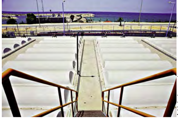
Ashkelon's seawater reverse osmosis plant
